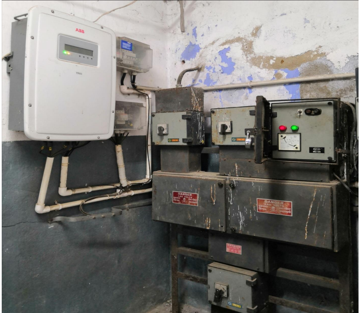
Picture of Net Meter for Solar PV Generation System
